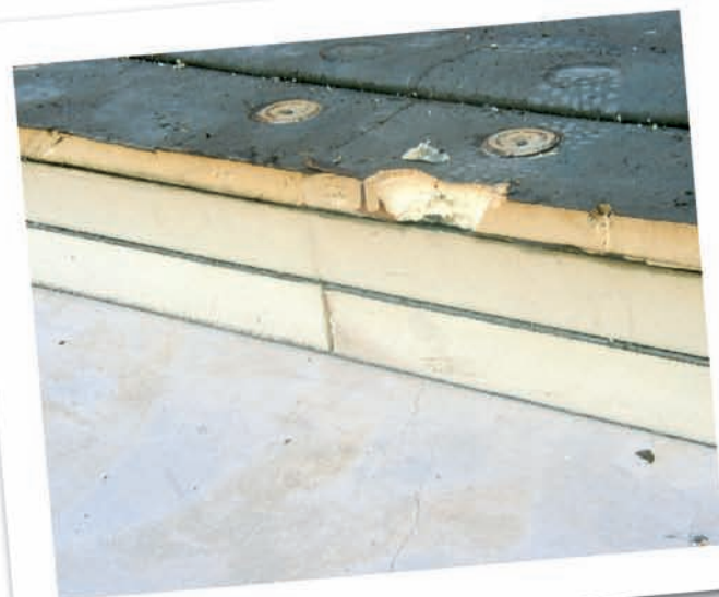
Figure 5: Damaged oxidized polyisocyanurate.
