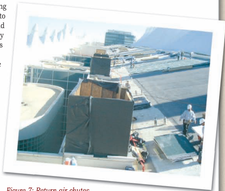
Figure 7: Return air chutes.
