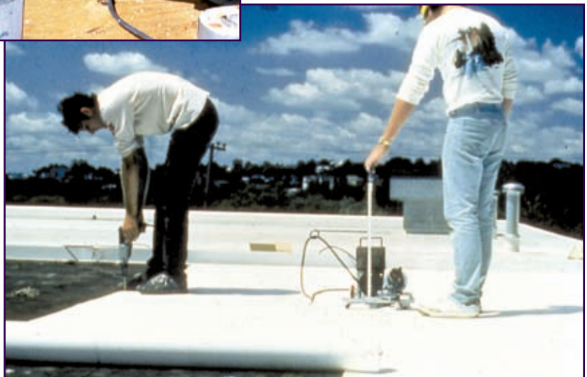
Figure 14: Lead weights have been stacked on this seam welder to improve CPE seam fusion.
