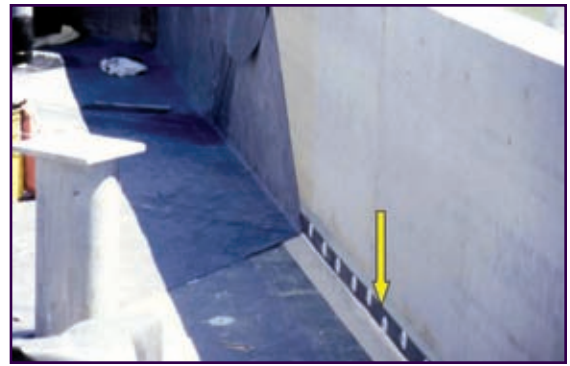
Figure 19: Edge restraint strips have reduced the tendency towards shrinkage and tenting of single-ply membranes.
