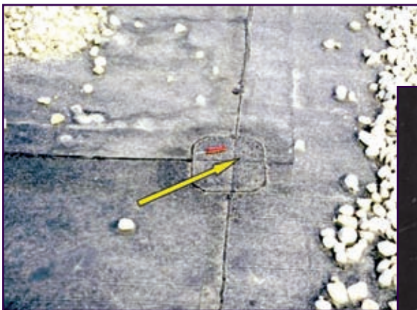
Figure 21: In retrofitting older EPDM roofs, all flashings are generally replaced and target pieces are added at all critical joints.
