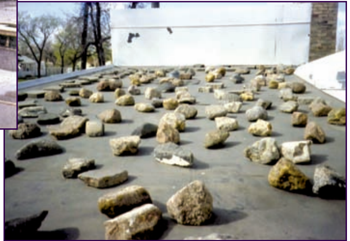
Figure 24: King-sized ballast on this roof!
