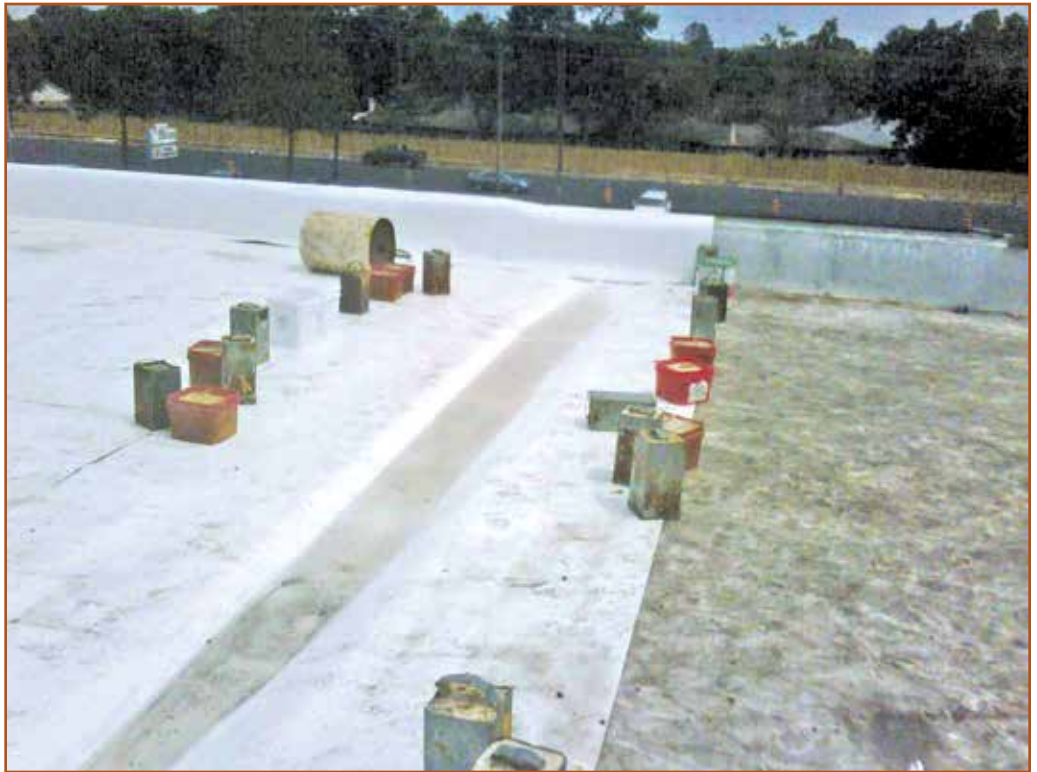
Photo 4 – Water accumulation on depression at tie-in.
