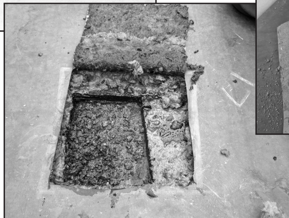
Photo 2 – Moisture-damaged fiberboard cover board.
