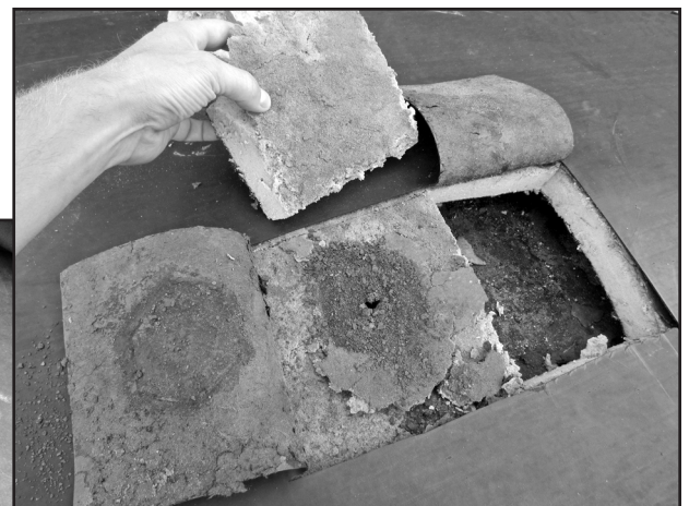
Photo 3 – Corrosion of roofing fastener.
