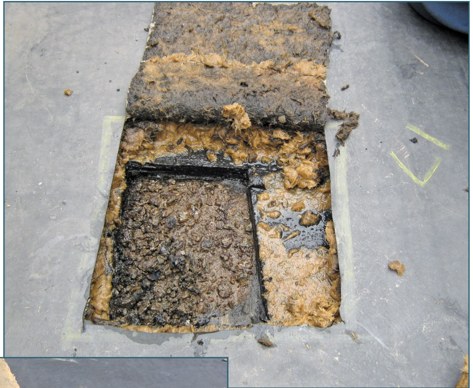
Photo 2 – Moisture-damaged fiberboard cover board.
