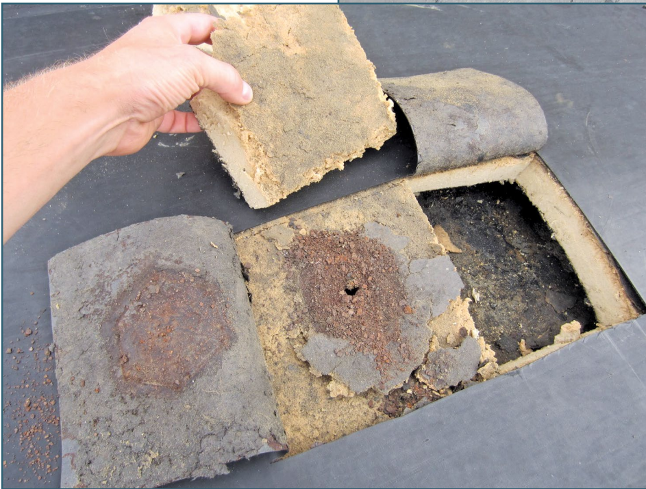
Photo 3 – Corrosion of roofing fastener.
